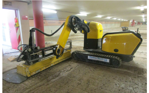
High pressure water jets were employed to remove the concrete containing chloride (Photo: AMP)
