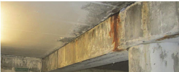
Reinforced concrete beam before restoration
