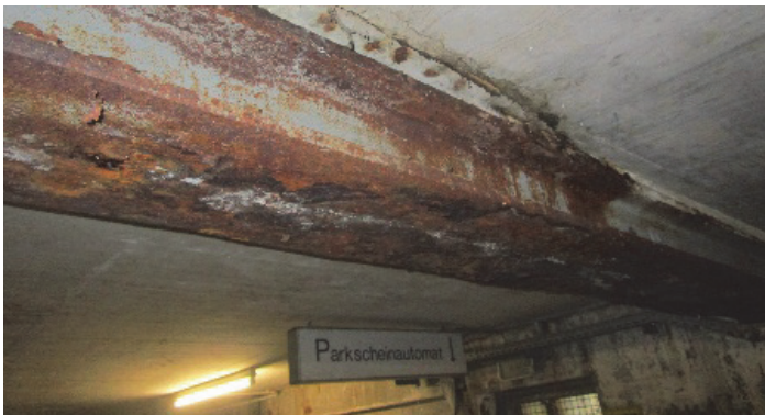
Corroding steel beam before restoration
